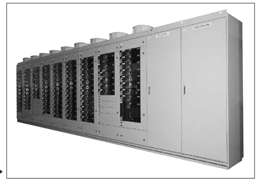
Photo 1 IGBT PWM inverter for processing line ▶
