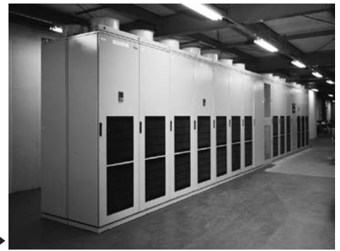
Photo 6 IGBT PWM inverter for mill drive ▶
